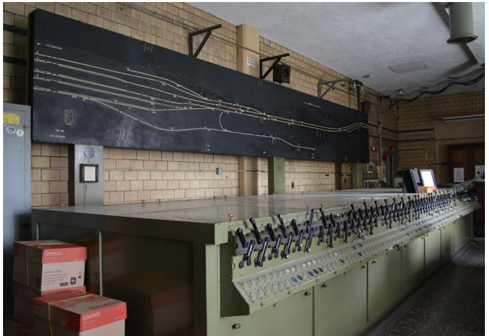
State Tower, housed on the main floor of the Harrisburg Transportation Center's 1936 addition houses this Model 14, Union Switch and Signal unit. The same equipment is used to control the interlockings at other points in the system from other nearby interlocking towers, including the Harris Tower.
