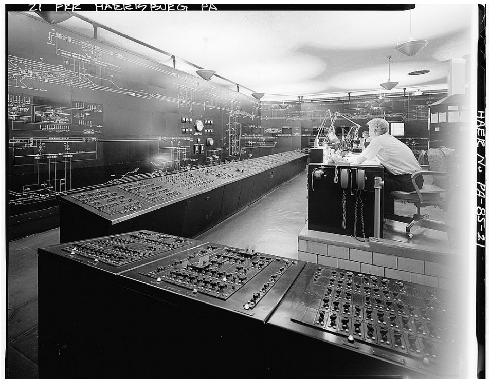
The Power Director's Office, seen in operation in this 1986 photograph, was the point of control for the system in the area around Harrisburg from its inception in the 1930s through c. 2013.
